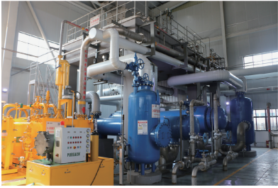
(a) 离心压缩机物理平台 (a) Centrifugal compressor physics platform
